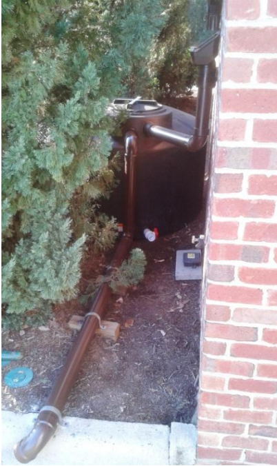
Figure 9 Cary Fire Station #1 Cistern
