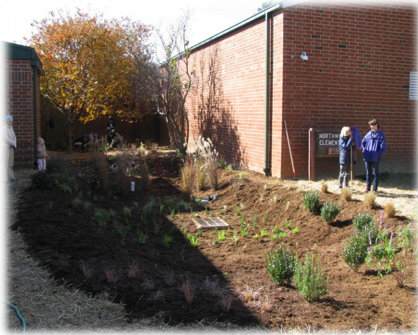
Figure 8 Northwoods Elementary courtyard bioretention after
