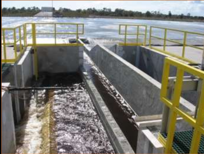
Harvested algae is conveyed by the water via a concrete flume to a centralized recovery facility.
