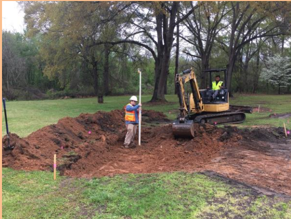
City of Raleigh Stormwater cost share helped pay for the St. Ambrose rain garden, shown under construction.
