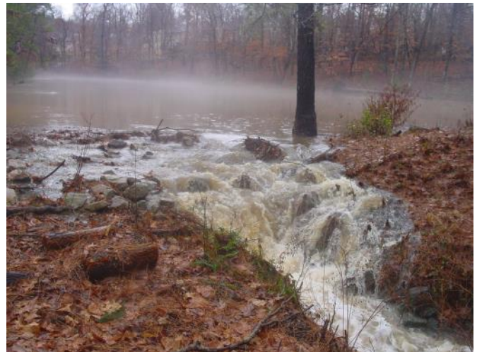
One of the Beechtree pond outfalls after rain (Amin Davis)
