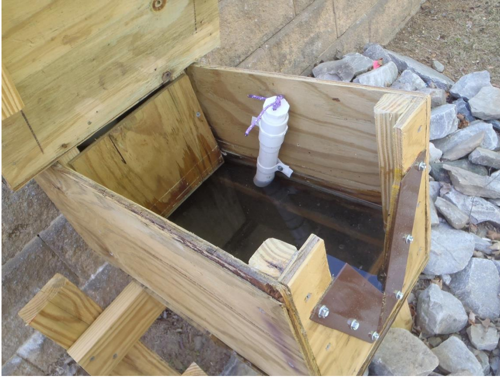
Figure 1. Weir box located at DT 3 inch inlet from roof.
