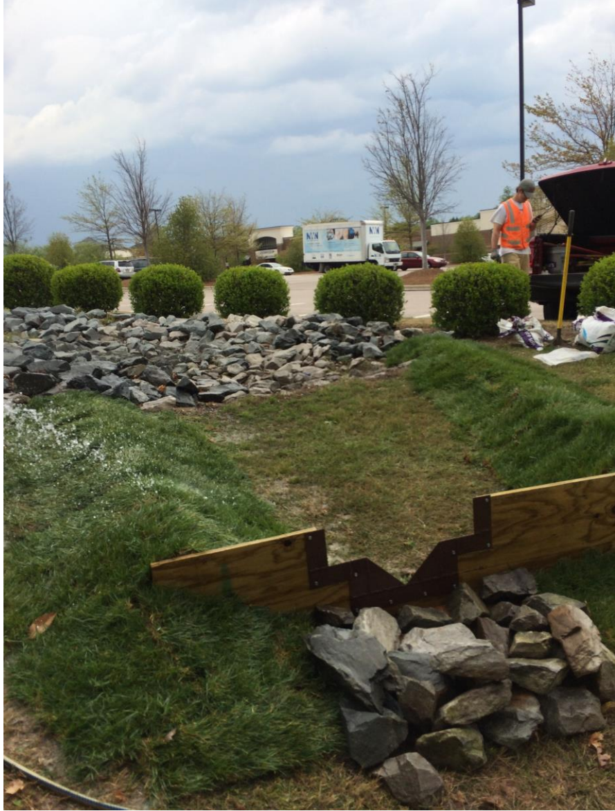
Figure 3. Compound weir installed to monitor parking lot runoff at DT.
