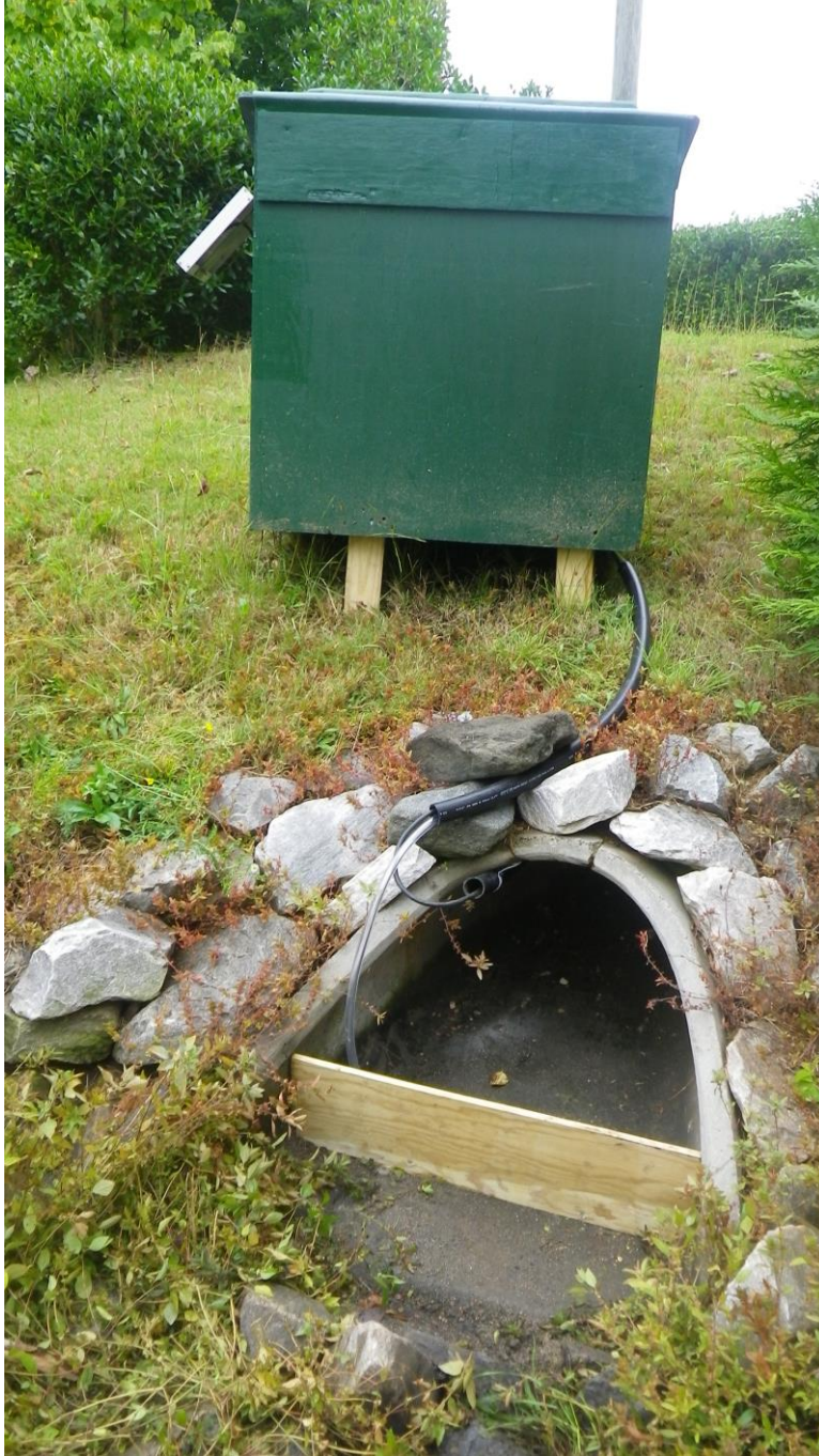
Figure 2. Inlet apron from 15-inch RCP at AAuto with sample box.
