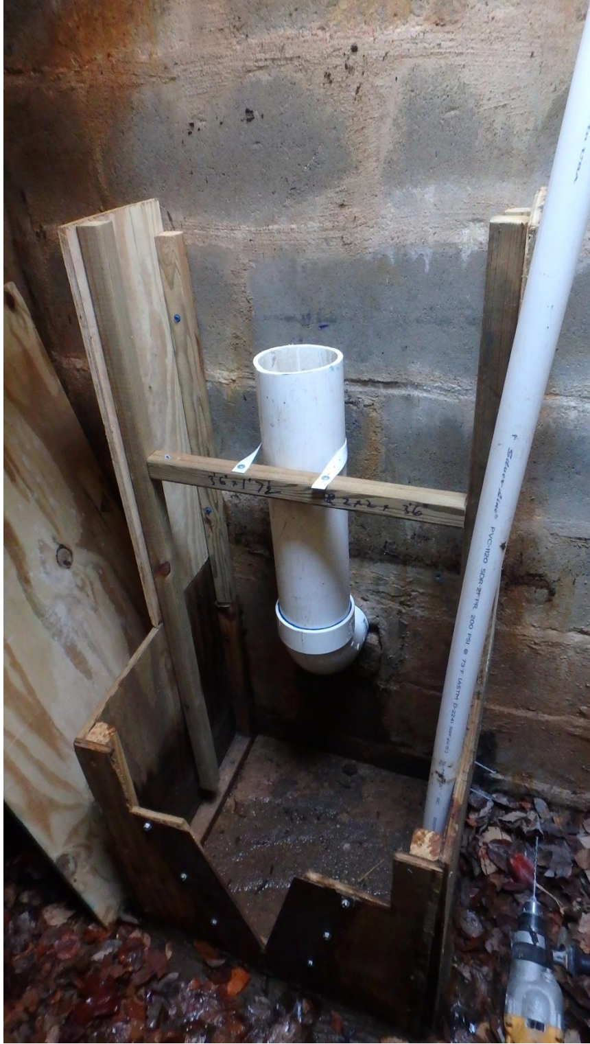
Figure 6. Post-retrofit elevated underdrain at DT using a simple upturned elbow.
